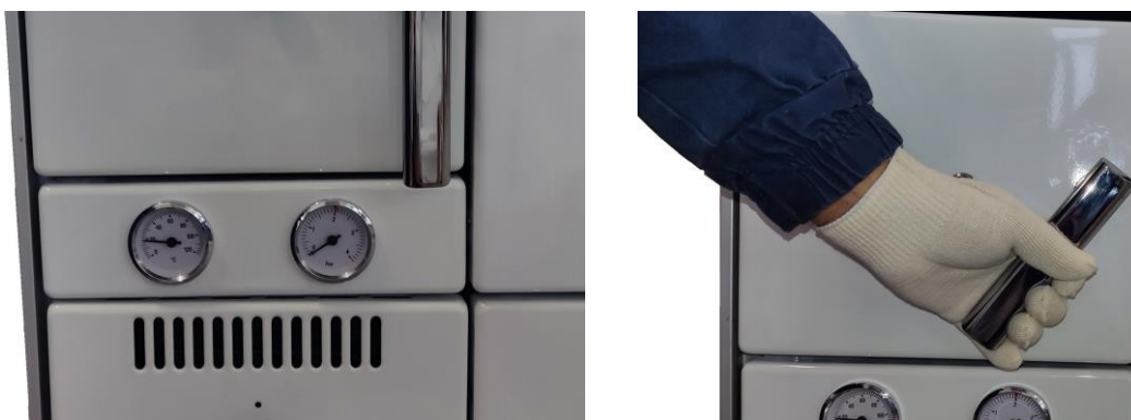
Figure 8. Boiler thermometer and pressure gauge, and operation of the combustion thermostat knob.
